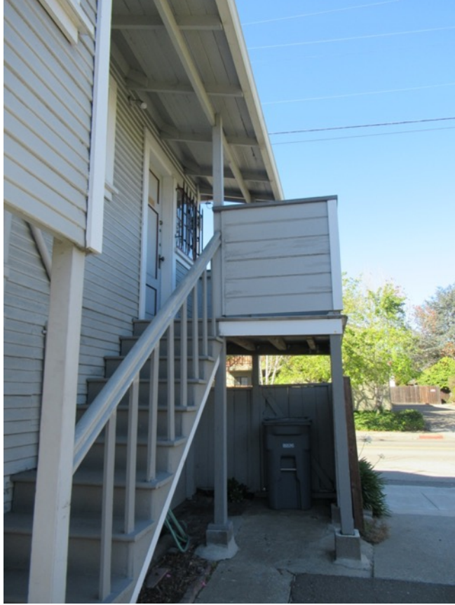
444 Kearney Street, detail of the staircase on the east façade, view north (Forget Me Not History, February 2022).
