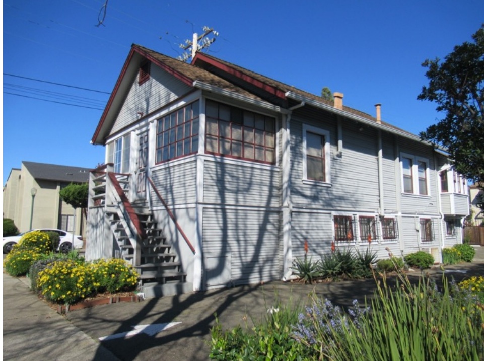
444 Kearney Street, west and south façades, view north (Forget Me Not History, February 2022).
