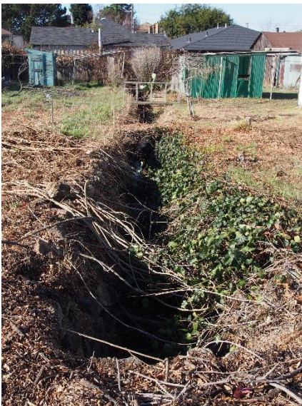
Clearing up to creek and debris in creek, no erosion protection
