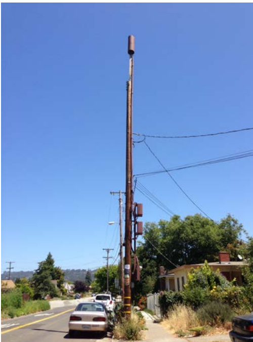
DAS node near 1215 Santa Fe Avenue, Berkeley
