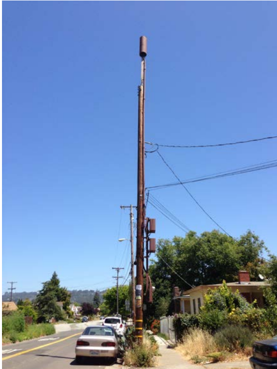
DAS node near 1215 Santa Fe Avenue, Berkeley
