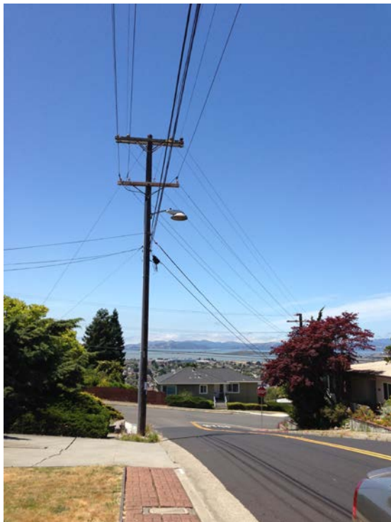
Existing pole near 7800 Eureka Avenue.
