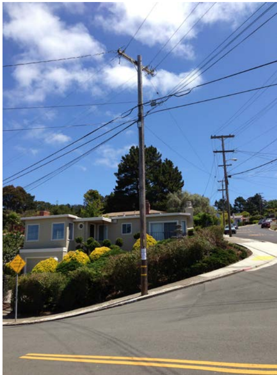
Existing Pole near 906 Galvin Drive.
