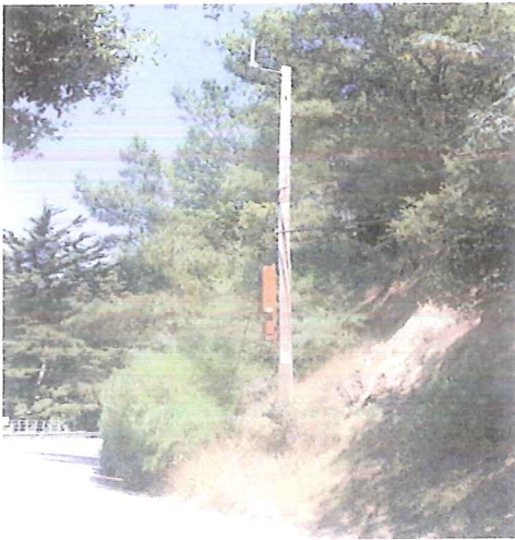
Half-mast DAS antenna at 6655 Snake Road, Oakland
