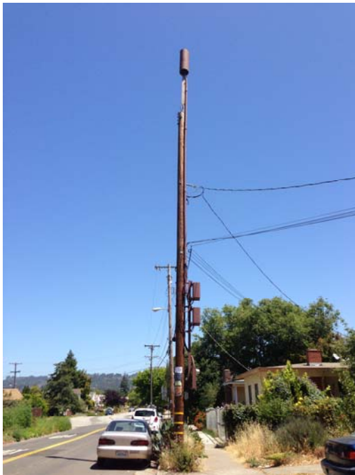
DAS node near 1215 Santa Fe Avenue, Berkeley
