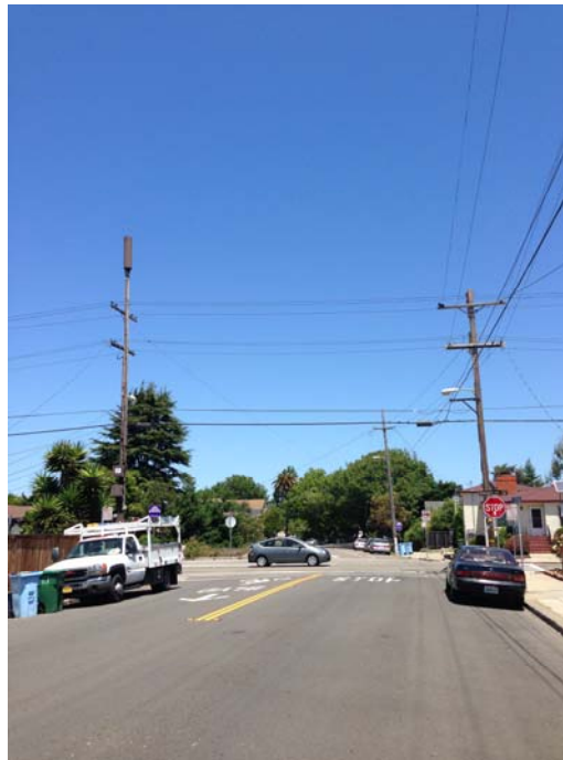
DAS node near Dwight Way and California Street, Berkeley
